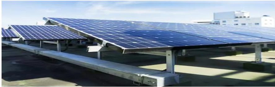
Fig. 1. Solar Panels are installed in the rooftop of the building.
